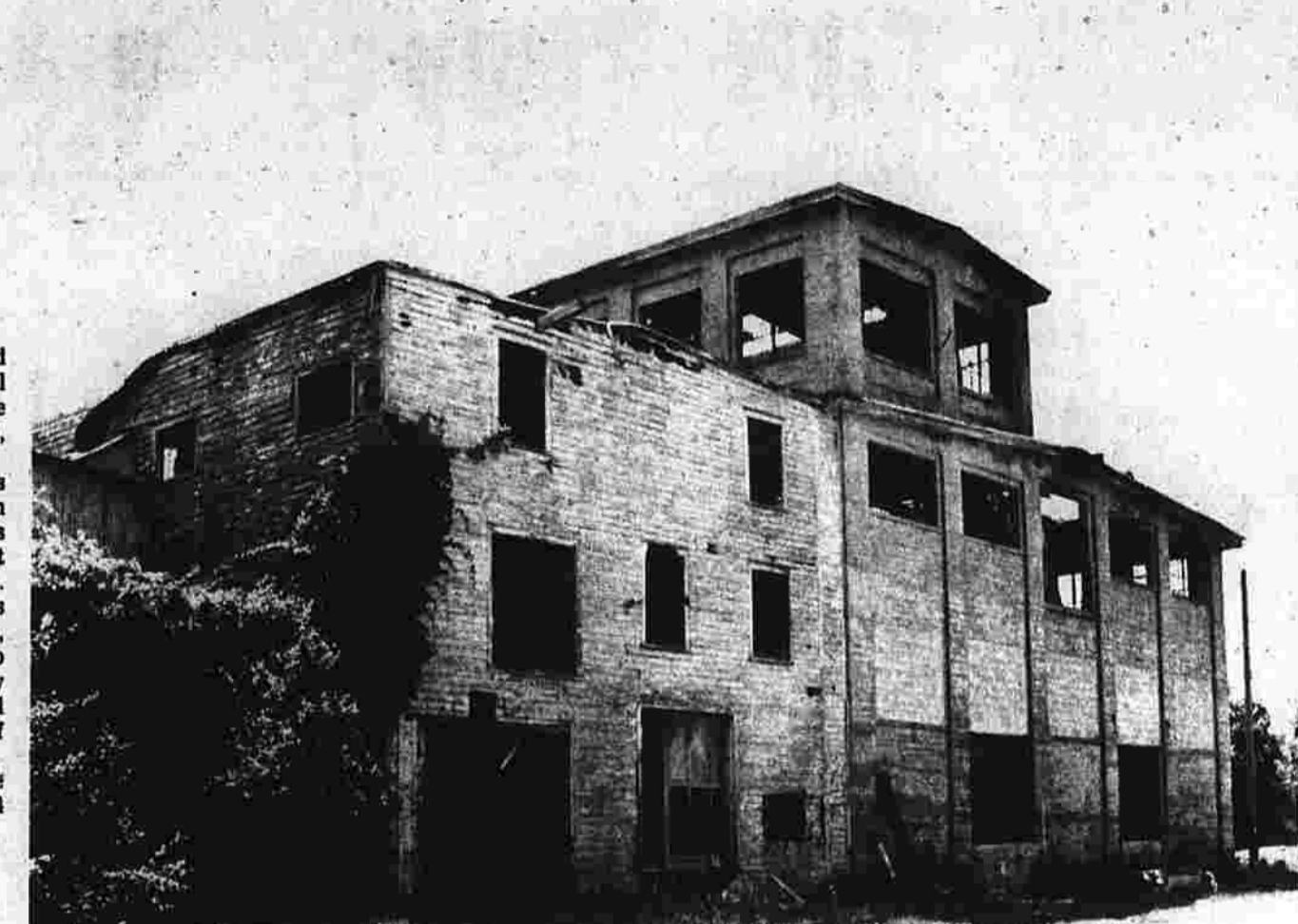
Six Months After Fire A view of the north side of the warehouse off Hillard St. One of the buildings in the former Bon Ami Manufacturing Co. complex, looks about the same as it did just after the Jan. 8 fire which gutted the structure.
